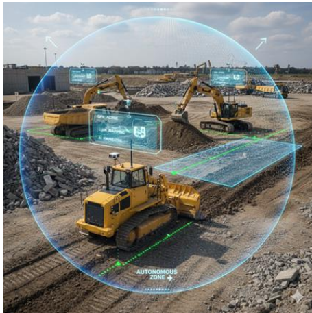
Figure 1 – Autonomous dozers, excavators, or haul trucks operating on a construction site (with GPS, LiDAR, and AI navigation overlays)
